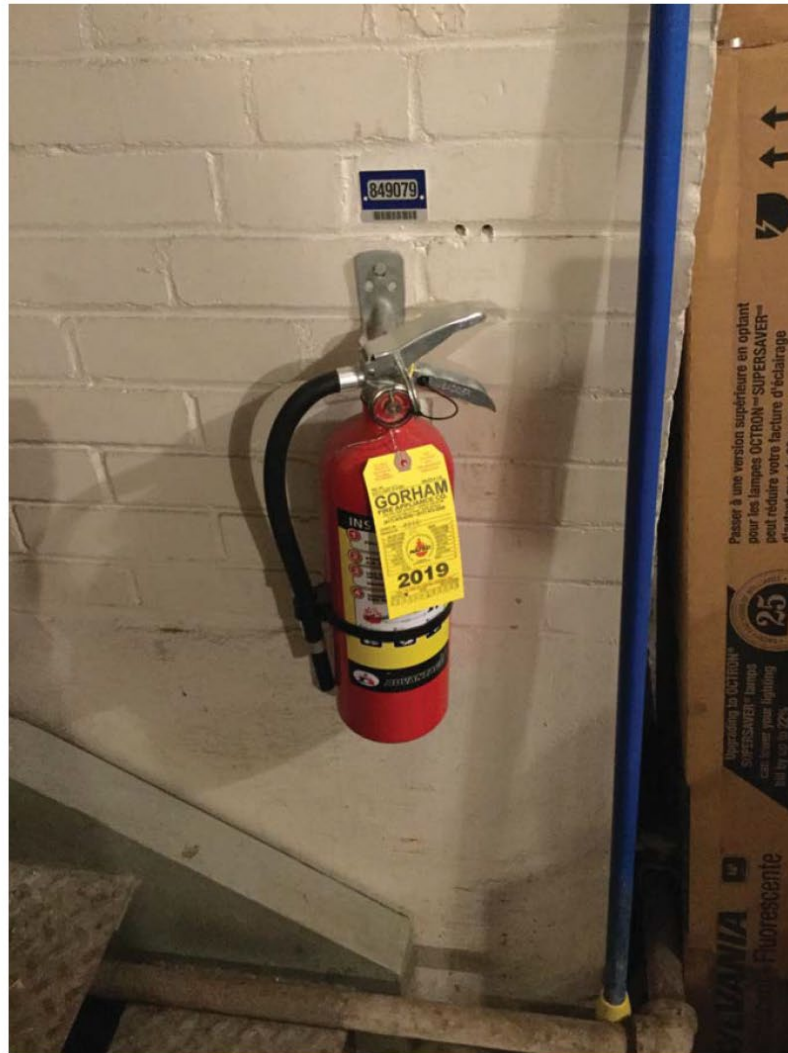
Equipment ID#: 849079 | Description: FIRE EXTINGUISHER
