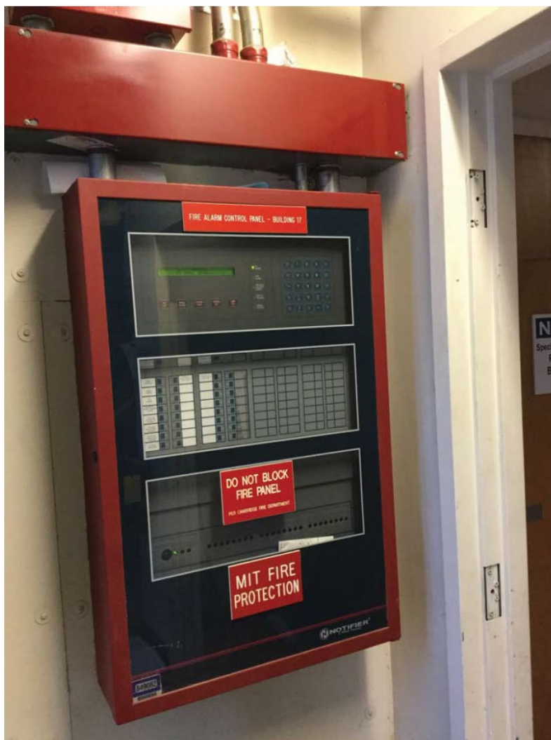
Equipment ID#: 849082 | Description: PANEL CONTROL FIRE
