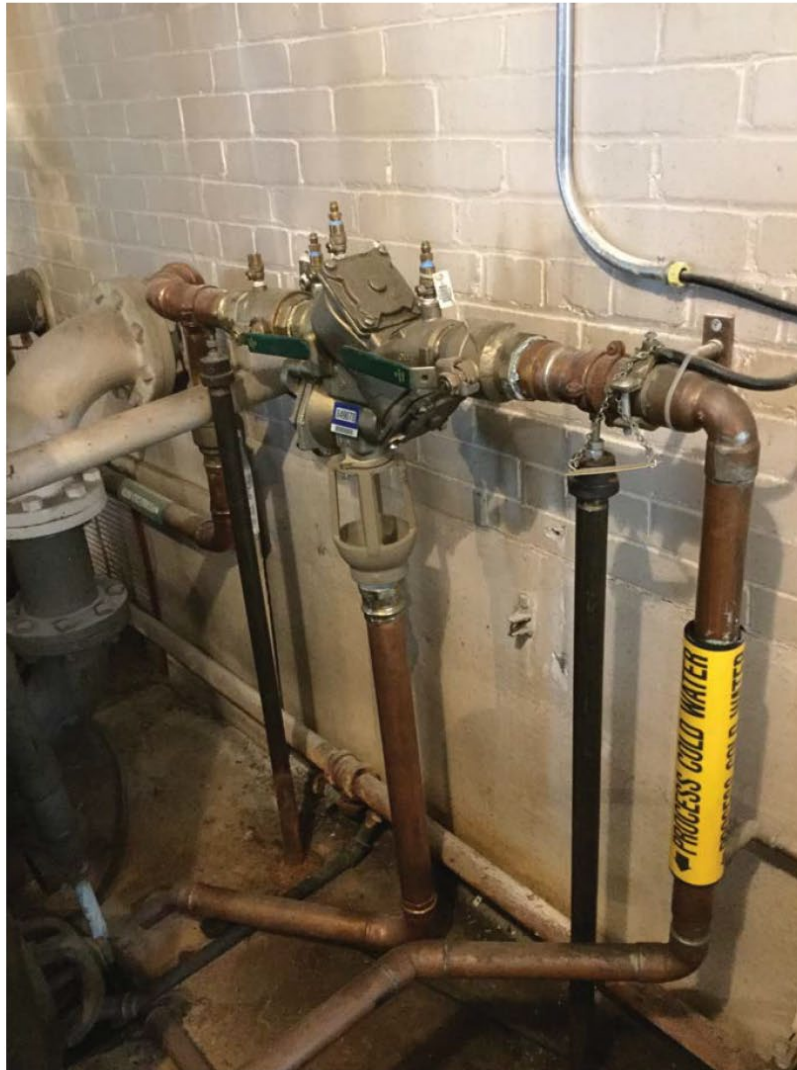
Equipment ID#: 849078 | Description: BACKFLOW PREVENTER
